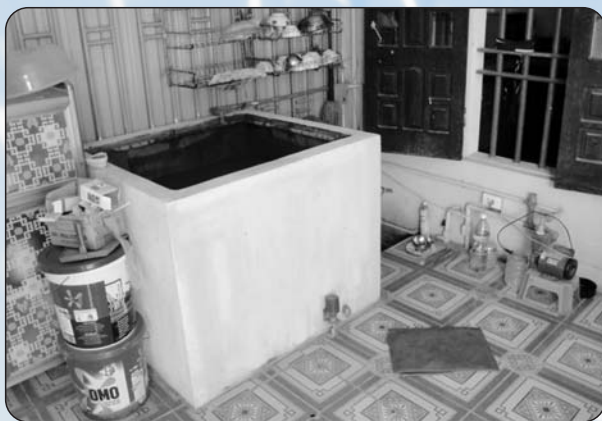
Simple filter system installed in a private household in the south of Nam Dinh province filtering extracted groundwater to improve drinking water quality.
